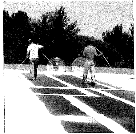
Apply Acrylic base coat with fabric embedded in base coat on entire roof
